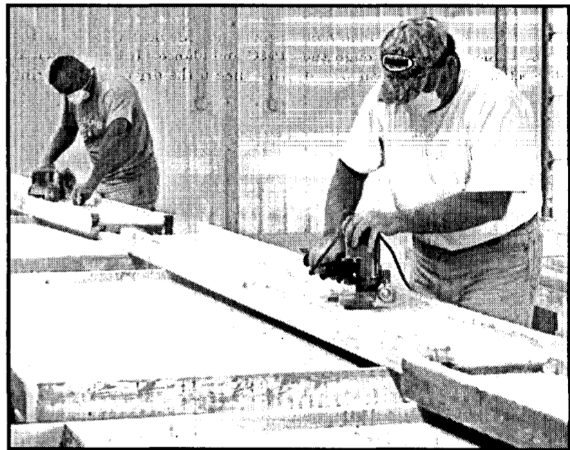
Volunteers work on sanding and painting the vendor booths in the Commercial Building on the fairgrounds.
